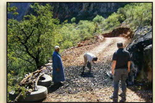
An example of the road improvements. A tyre fire was burned overnight to damage the rock to facilitate breaking it to widen the road into the Tamza Valley. The protagonists were happy to drag the remnants aside so we could drive through – quickly before our tyres melted on the hot gravel, ashes and tyre wires!
